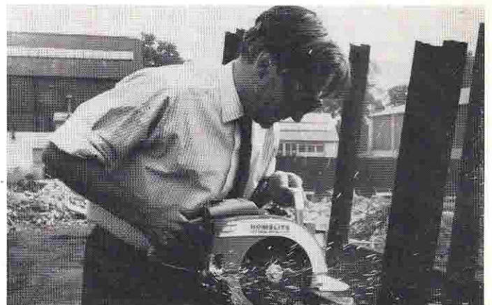
Trojan Works, Homelite's distributor in Great Britain, sent this picture out with a publicity release about the XL-100 circular saw. It shows a man using "the new petrol-driven Homelite XL-100 circular saw to cut a four inch steel girder on a demolition site."
