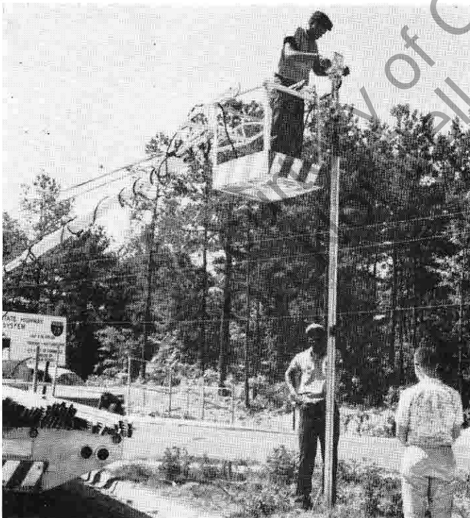
Riding high, wide and handy, an employee of Warning Lights and Systems, Inc., of Atlanta, Georgia, drives in a post on Interstate Highway #20. He clips his Homelite-Bosch Paving Breaker to the post, drives it in then lifts the PB back to support arms on the basket and is carried on to the next location. Another way in which Homelite serves to make a hard job easy.
