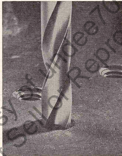
Fig. CS51 — Drill out the old threads or broken stud, using drill size recommended in instruction sheet which comes with kit. Drill all the way through an open hole or all the way to bottom of a blind hole, making sure hole is straight and that centerline is not moved in drilling process.
