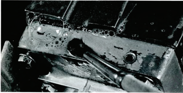
SOAP BUBBLES DISCLOSE LEAK NEAR LOOSE SCREW.
